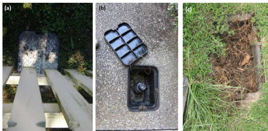
Figure 3: Examples of unsuitable water meter boxes.
