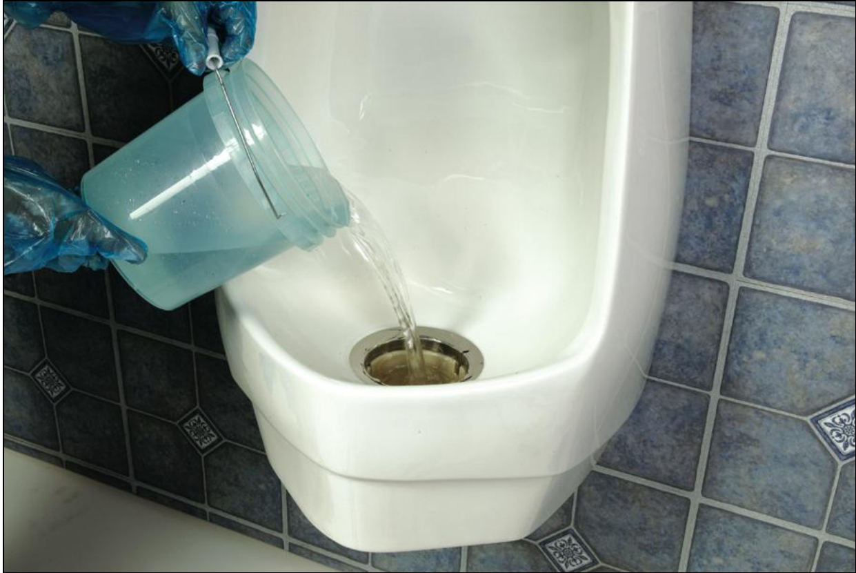
Figure 17. Pouring water into a non-water urinal system to clean drain pipes.
