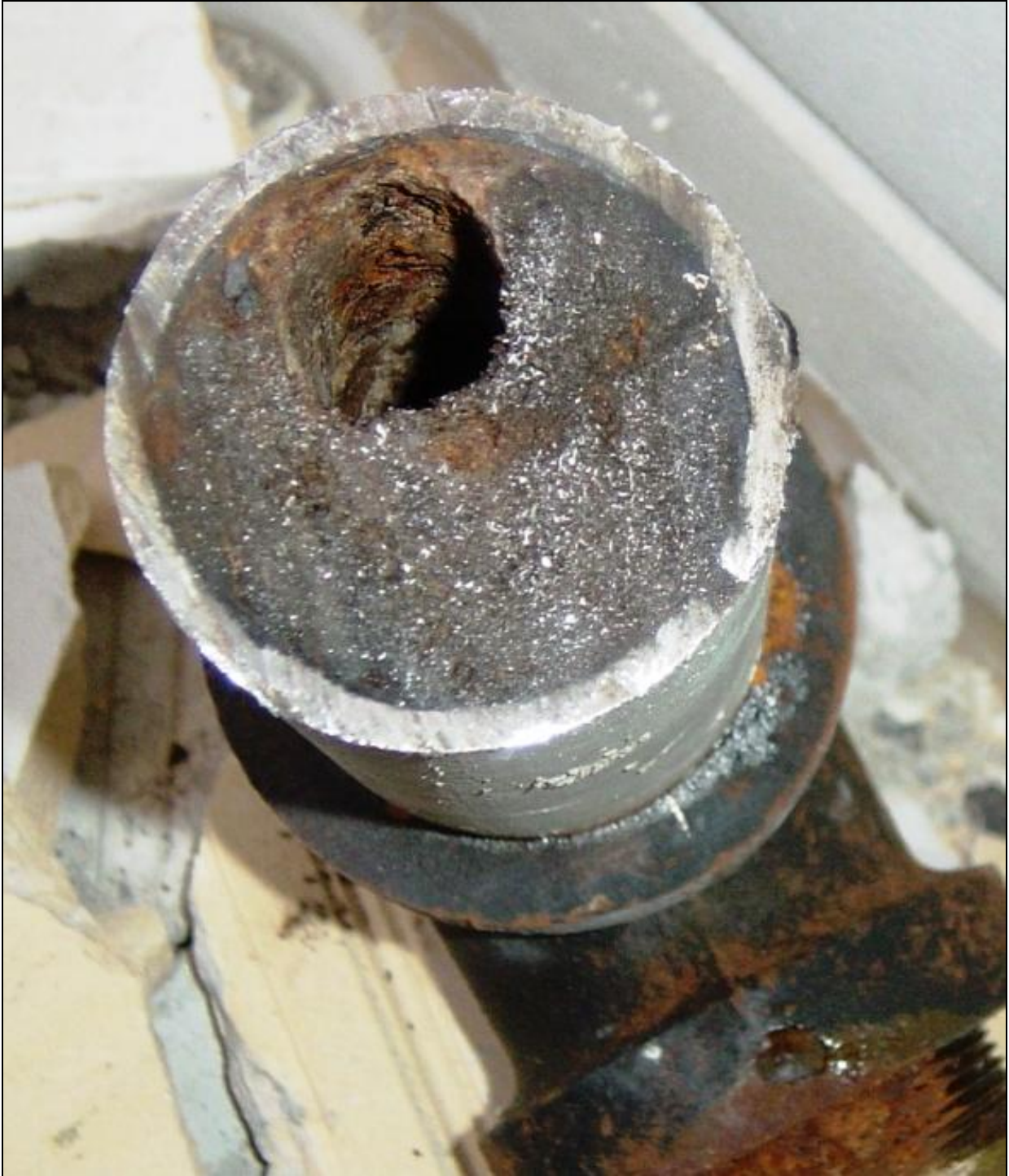
Figure 9. Drain pipe for water-flushing urinal at Fort Bliss in El Paso County, Texas, removed after 8 years of service.
