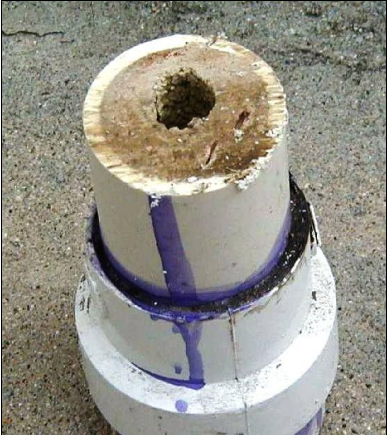
Figure 12. Vertical stack drain pipe for water-flushing urinal at Lackland Air Force Base in San Antonio, Texas, removed after 24 months of service.
