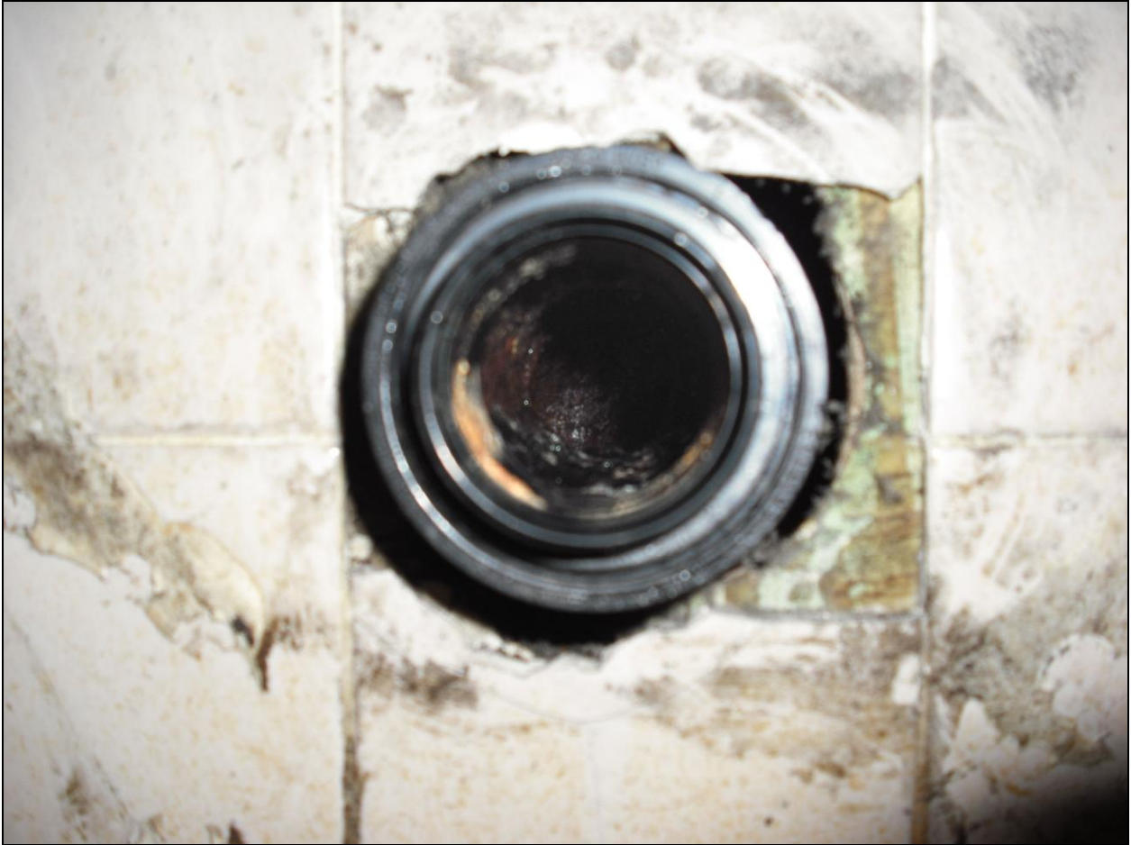
Figure 27. Close-up detail of the horizontal pipe nipple immediately after removing the non-water urinal, after seven years of continuous operation.
