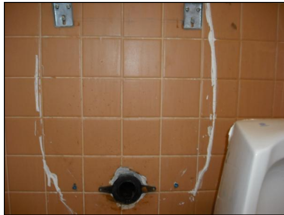
Figure 38. Non-water urinal removed September 2008 for drain line inspection.
