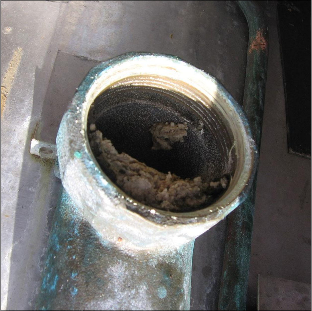
Figure 14. Urinal outlet for water-flushing urinal at Los Angeles County Beaches, removed after 3 years of service.
