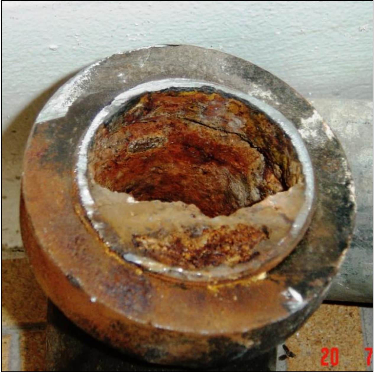
Figure 10. Drain pipe for water-flushing urinal at Fort Bliss in El Paso County, Texas, removed after 8 years of service.
