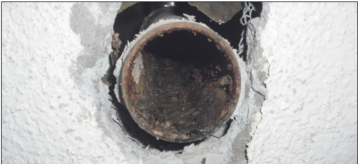
Figure 35. Close-up detail of the horizontal pipe nipple immediately after removing the non-water urinal, after six years of continuous operation.
