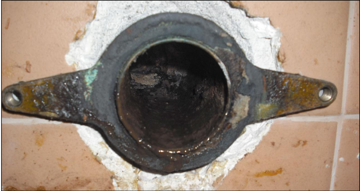
Figure 39. Close-up detail of the horizontal pipe nipple immediately after removing the non-water urinal, after five years of continuous operation.
