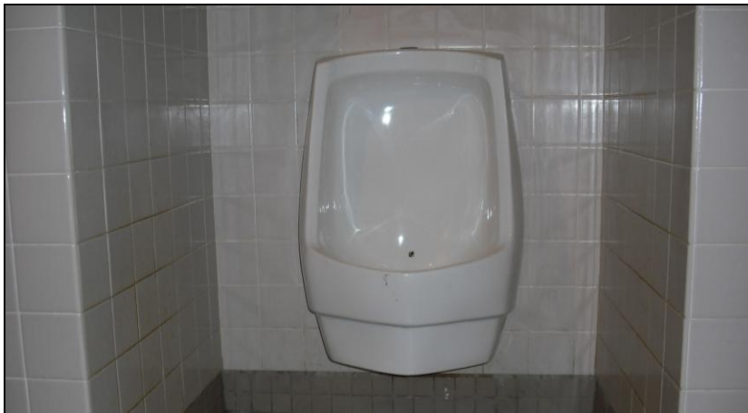
Figure 25. Non-water urinal installed as part of city rebate program in 2001. Typical installation on the fourth floor of this 11-story office building.
