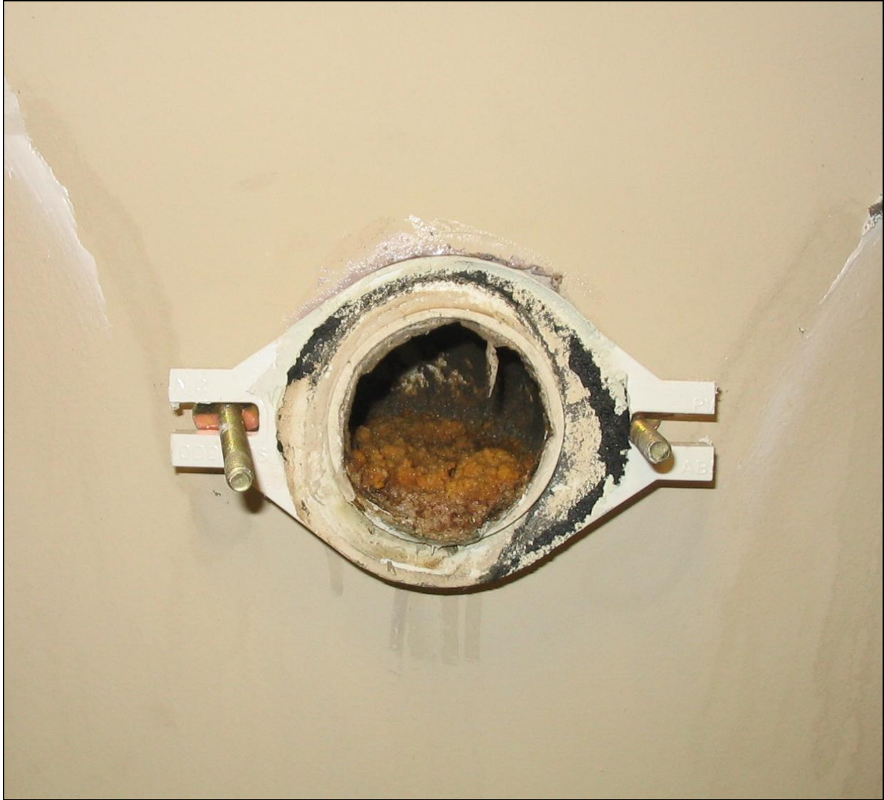
Figure 15. Horizontal pipe nipple/drain connection in 2005 after removing a water flushing urinal that had been in operation for less than five years at CPR in Grand Rapids, Michigan.
