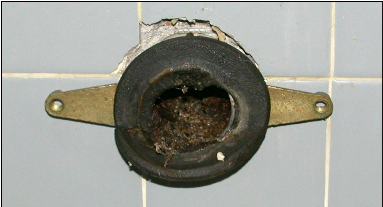
Figure 21. St. Louis County Health Department, 2003. Drain line after removing water flushing urinal that had been in service for 21 months.
