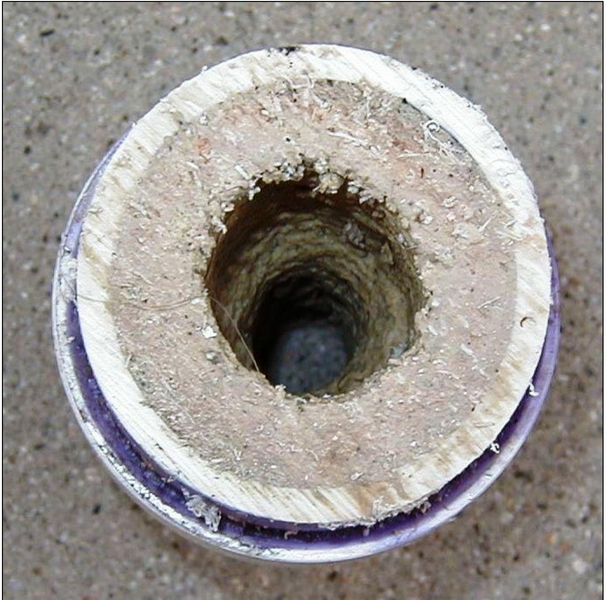
Figure 13. Vertical stack drain pipe for water-flushing urinal at Lackland Air Force Base in San Antonio, Texas, removed after 24 months of service.
