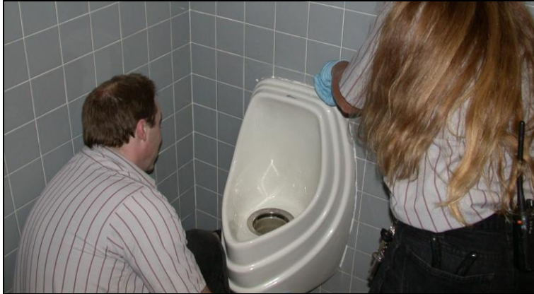
Figure 23. St. Louis County Health Department. Removing the Falcon Waterfree urinal to inspect the drain line after one year of continuous operation.
