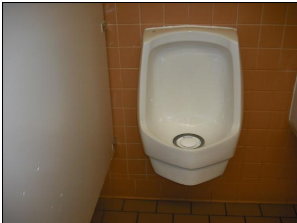
Figure 37. Original installation (retrofit of water-flushing urinal) took place in 2003.
