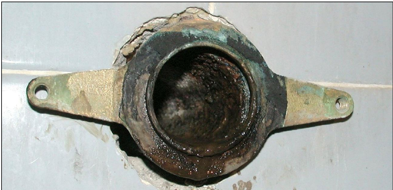
Figure 24. St. Louis County Health Department. Drain line immediately after removing the Falcon Waterfree urinal, after one year of continuous operation. The Falcon Waterfree urinal was reinstalled and continues to be in use at this location.
