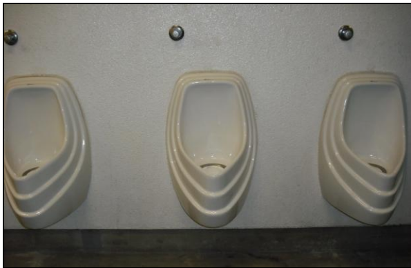
Figure 33. Original installation (retrofit of water-flushing urinal) took place in 2002.
