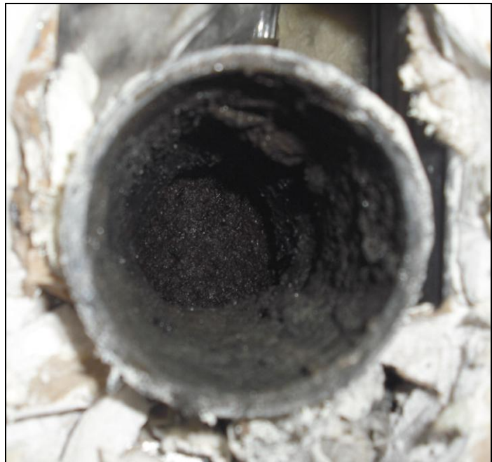
Figure 32. Close-up detail of the horizontal pipe nipple immediately after removing the non-water urinal, after five years of continuous operation.
