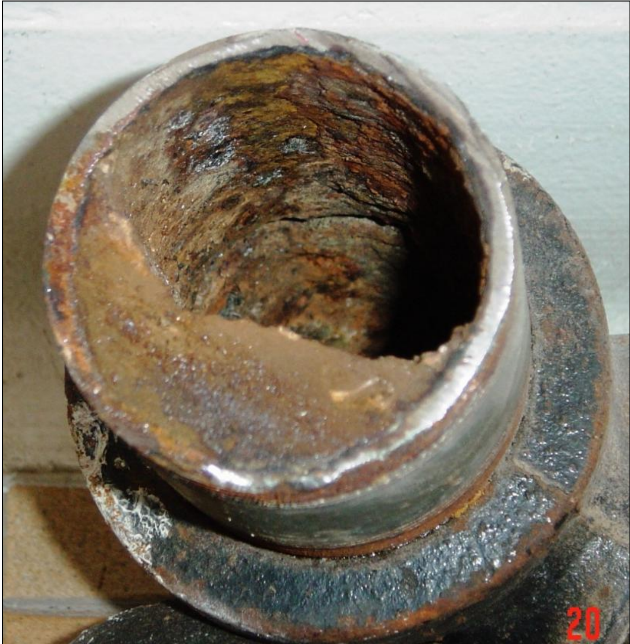
Figure 8. Drain pipe for water-flushing urinal at Fort Bliss in El Paso County, Texas, removed after 8 years of service.
